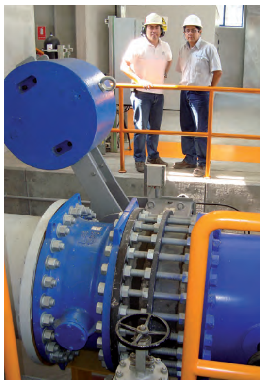
Mr Frank Maita and Daniel Ayulo in turbine house Huasahuasi I with one of the VAG EKN® Butterfly Valves with the huge lever and weight arm that quickly closes the pipe in the event of an emergency.
