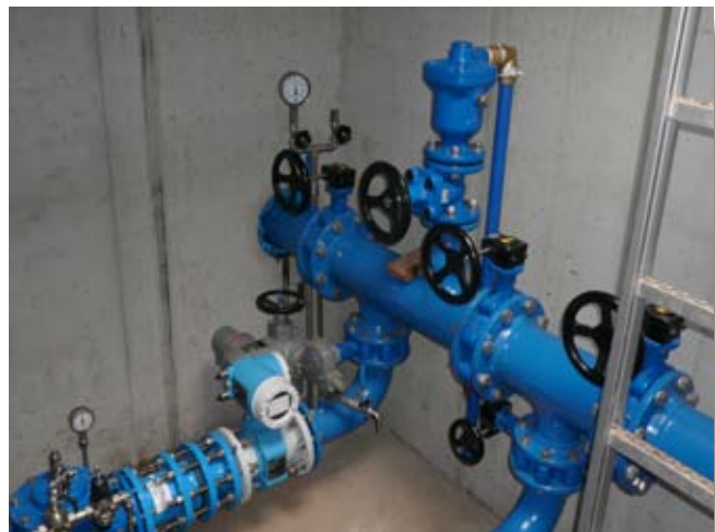
Outlet to the medium pressure zone with a VAG CEREX ® 300-L Butterfly Valve as a gear unit and a handwheel and an electric actuator
