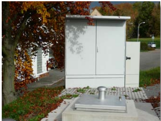
External view of the control cabinet
