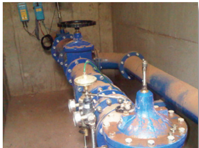
Valve installation chamber
