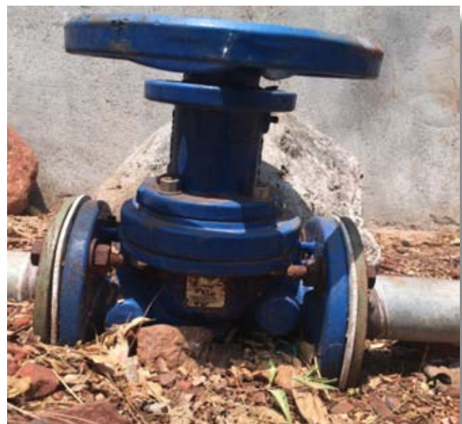
Installed VAG DURA Control Valve
