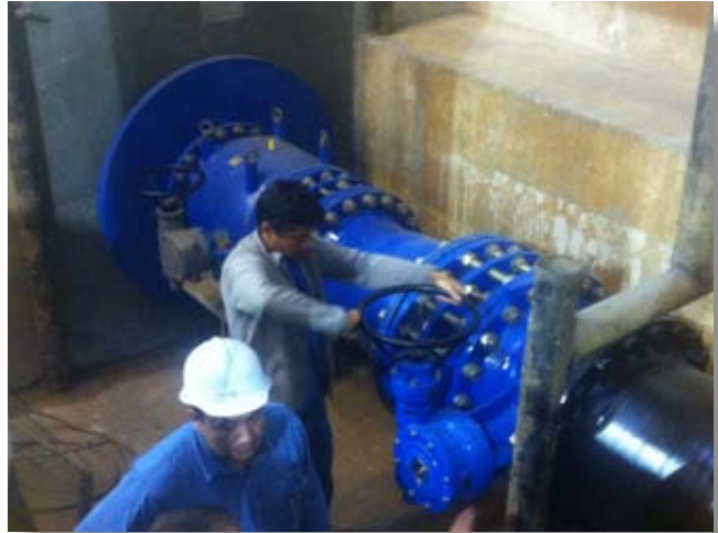
Built-in VAG RIKO ® Plunger Valve DN 500 next to a VAG EKN ® Butterfly Valve during inspection
