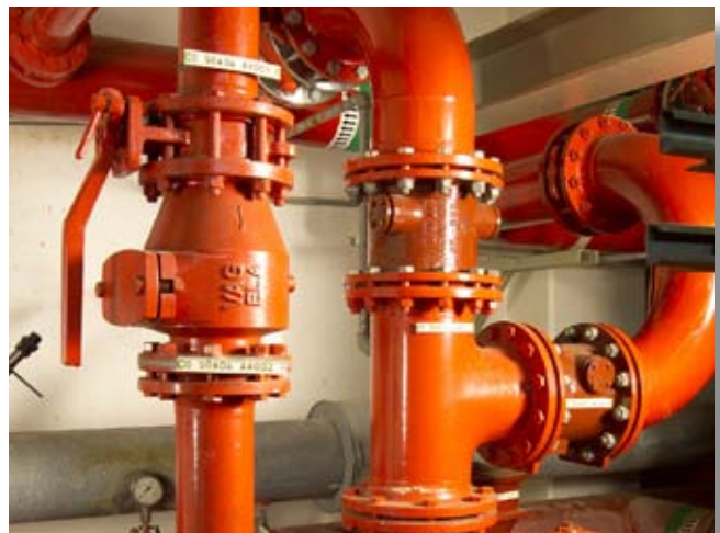
VAG RETO-STOP Non-Return Valve, VAG BETA® 200 Gate Valve and VAG SKR Slated-Seat Tilting-Disk Check Valve in the booster station of the fire-fighting system
