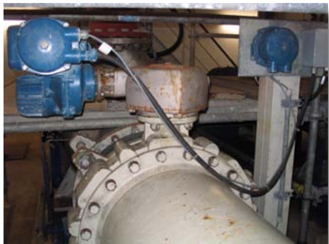
VAG CEREX® 300 Butterfly Valves and VAG SKR slanted seat tilting disk check valves in the associated intake structure
