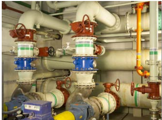
VAG EKN® Butterfly Valves, VAG EKO® plus Gate Valves and VAG SKR slanted seat tilting disk check valves in the pumping station of the fire-fighting system
