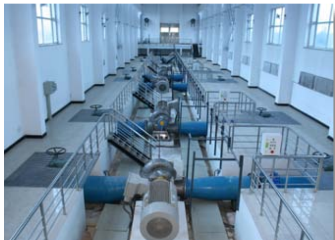
Station de pompage
