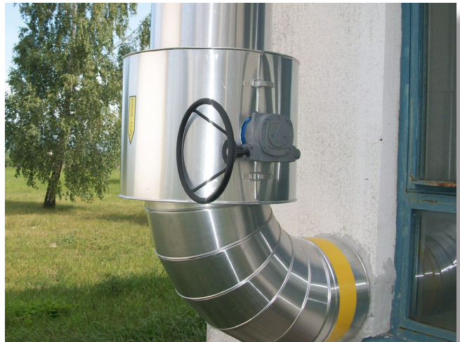
Isolated VAG EKN® Butterfly Valve in a gas-supply-pipeline
