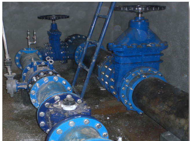
Valve installation chamber
