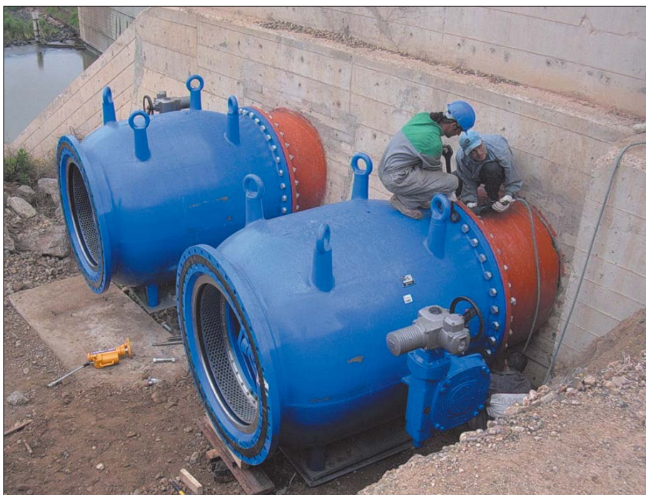
Fig. 8: Installation of two VAG Plunger valves DN 1200 at the Beni Bahdel dam, Algeria
