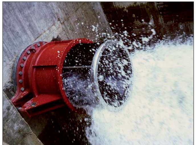
Fig. 5: VAG Hollow Jet valve DN 1000 in standard version installed in the bottom outlet of the dam La Copa, Colombia
