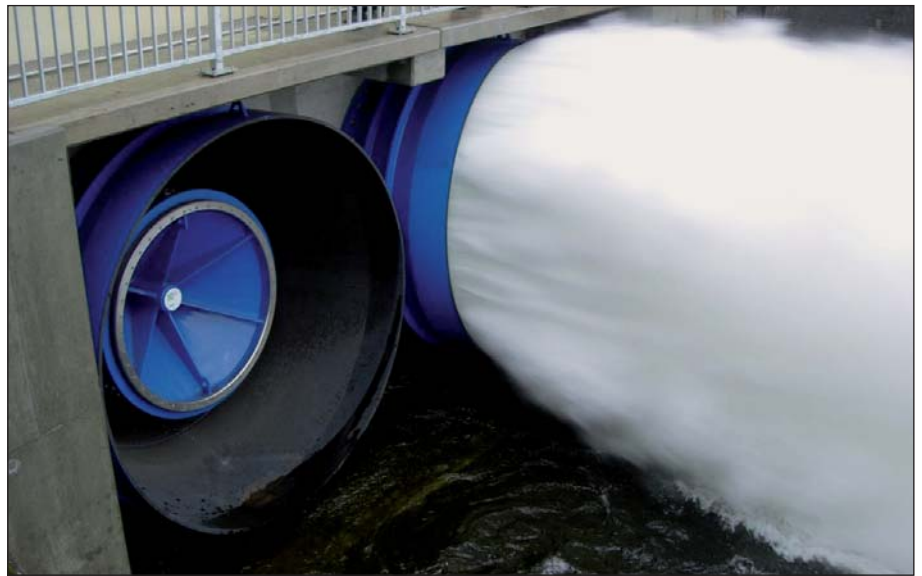
Fig. 6: 2 pc. VAG Hollow Jet valves DN 1800 with hood pipe (diameter 3600 mm) installed in the two bottom outlets of the RUR dam, Germany
