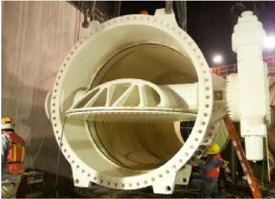
Picture: Butterfly valves in the factory hall, today...
